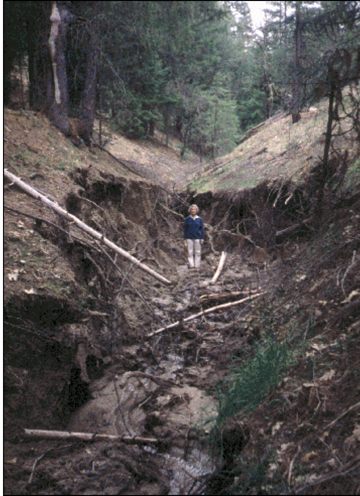
Figure 3-5. Gully Resulting from a Lack of Channel Protection.
