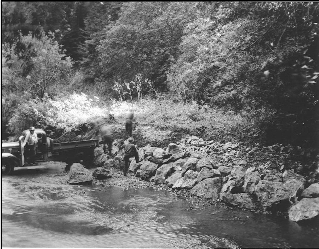
Figure 10. Equipment working in streambed during CCC riprap construction ca. 1937, note the bed and bank disturbance (from NPS Archives).
