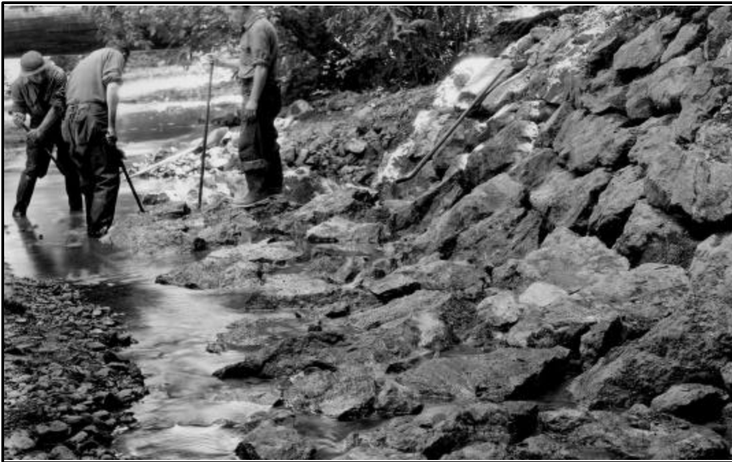
Figure 14. Rock riprap armoring the stream bank and extending into the channel as depicted in Figure 13 (from NPS Archives).
