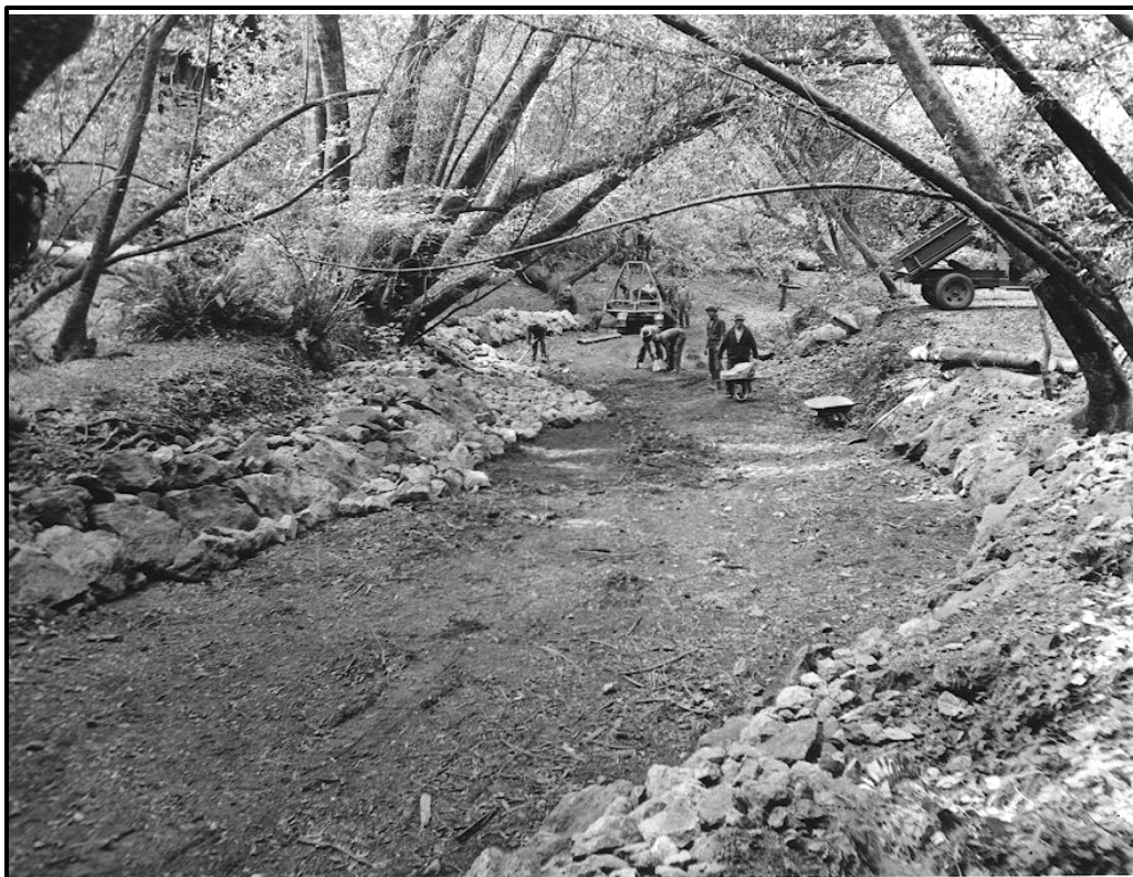
Figure 9. CCC workers installing rock riprap along the banks of Redwood Creek. Note the lack of bank vegetation and the truck on the bank, showing bank disturbance, also the machinery in the creek. ca. 1934 (from NPS Archives).
