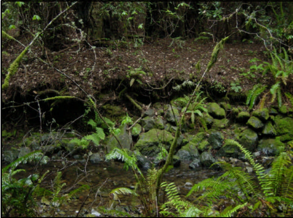
Figure 16. Downstream end of riprap section R9. Note the rock slumping into the channel and the bank scour on the left.
