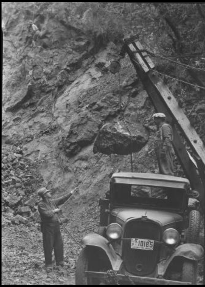
Figure 7. CCC workers loading rocks at the Kent quarry for riprap in Muir Woods ca. 1934 (from NPS Archives).
