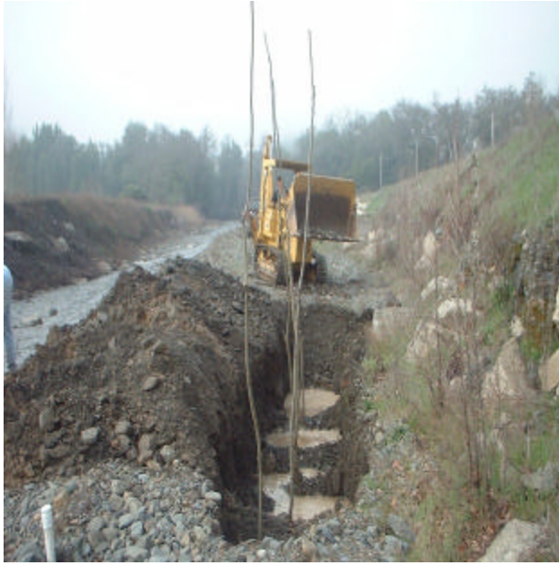
Restoration project on Morrison property included trenching of poles with a backhoe as well as revegetating with native species
