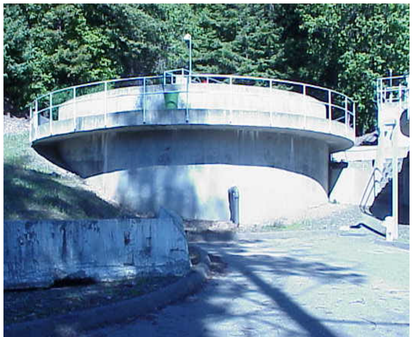
A third clarifier, similar to this one shown, will settle solids out of the liquid stream , allowing clarified effluent to move on to the tertiary filtration process.
