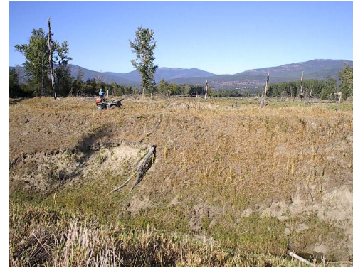
Unstable bank (downstream of primary cross-section) prior to placement of poplar matting
