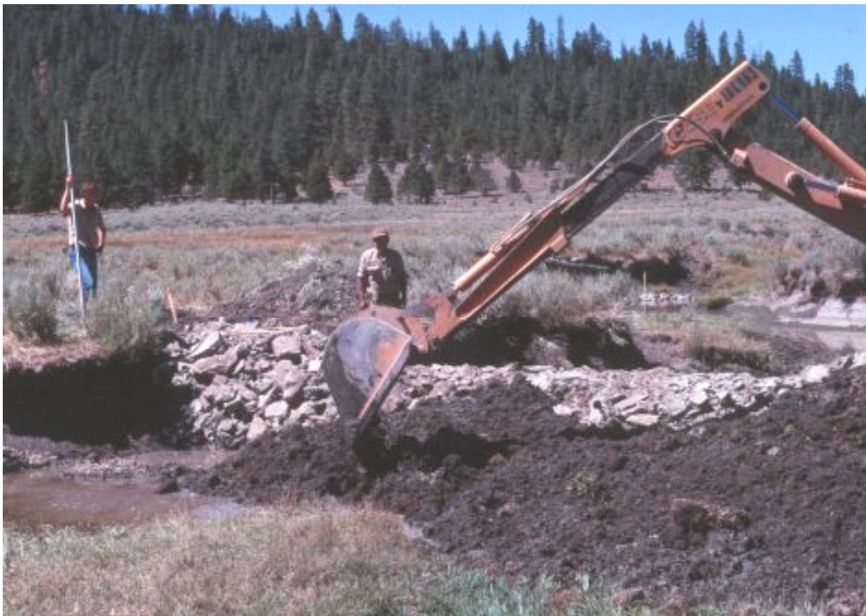
Photo 2. Rock check weir construction in creek channel under watchful eye of USDA Soil Conservation Service technician (holding survey rod), August 1985.
