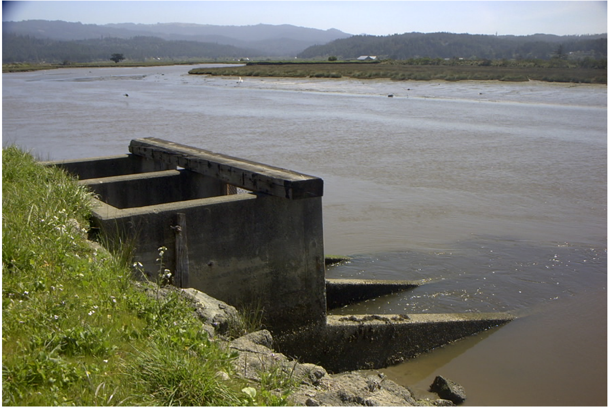
Figure 25. Tide gate separating Eureka Slough, Humboldt Bay, Humboldt County, California and the drainage ditch that parallels California State Highway 101. Eureka Slough is in the background.
