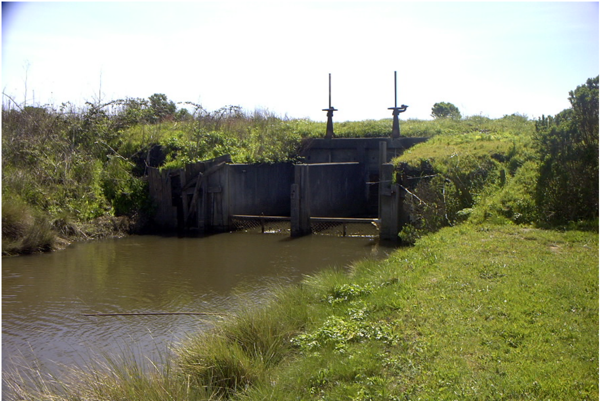
Figure 24. Tide gate separating Eureka Slough, Humboldt Bay, Humboldt County, California and the drainage ditch that parallels California State Highway 101. The drainage ditch is in the foreground.
